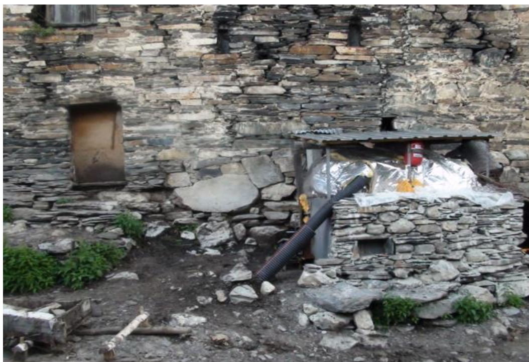
Thermophilic biogas digester installed in Ushguli
